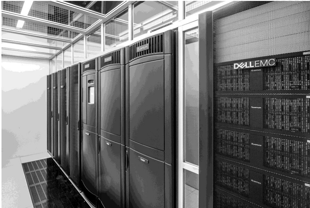
Figure 6 One of the adwäisEO server room hosting the CCI+ SSS processing system
